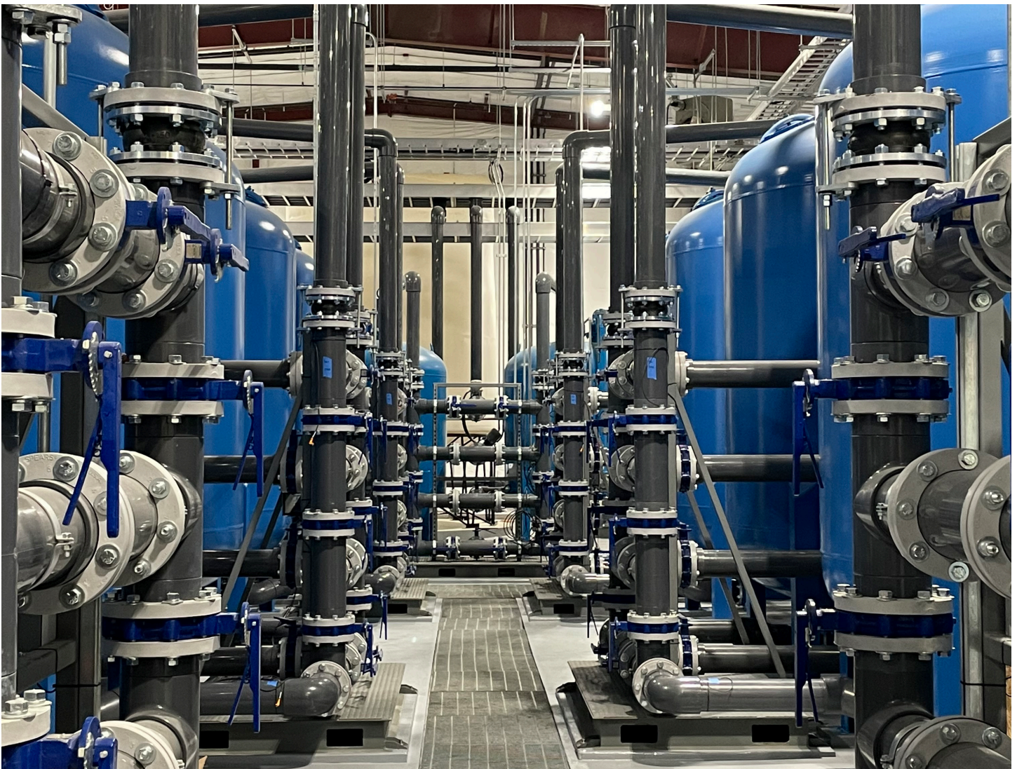
Granulated Activated Carbon (GAC) treatment vessels for the GETS
